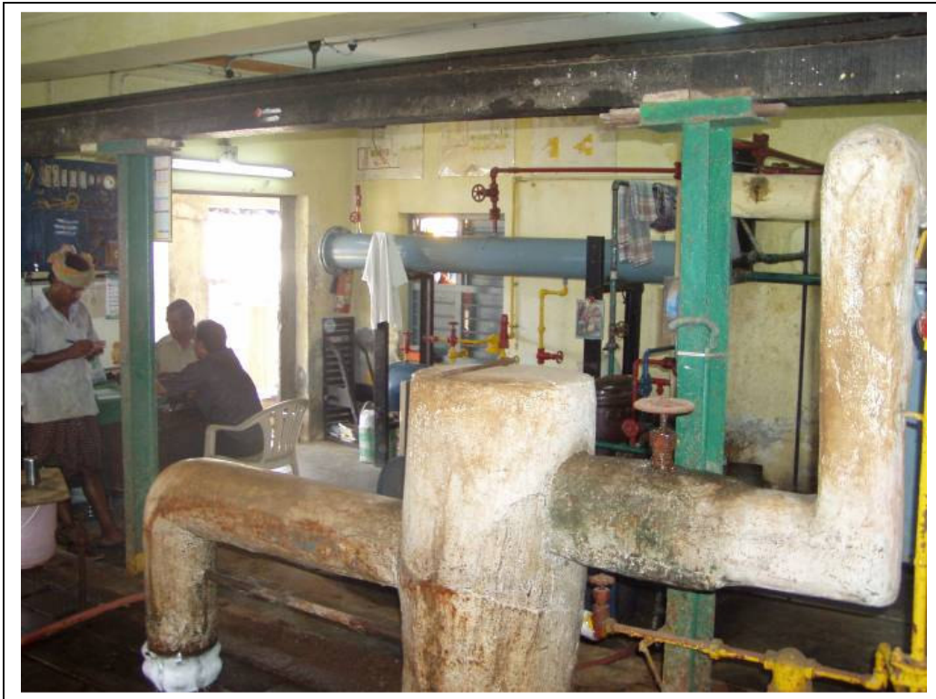
Govt. Ice Plant at Big Market, Puducherry
